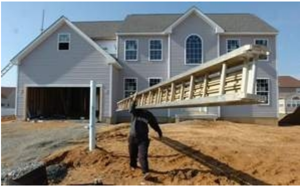
Work is under way on this new home at 125 Needham Dr. in Brenford Woods, near Smyrna. The community is one of the state's few bright spots in residential construction. / The News Journal/BOB HERBERT
